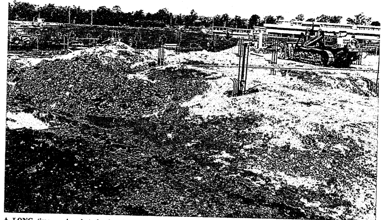
A LONG time coming, but the foundations are laid for the $1.8 million District Headquarters at Oxley. The new station is expected to be officially opened in the 1982-83 financial year.
