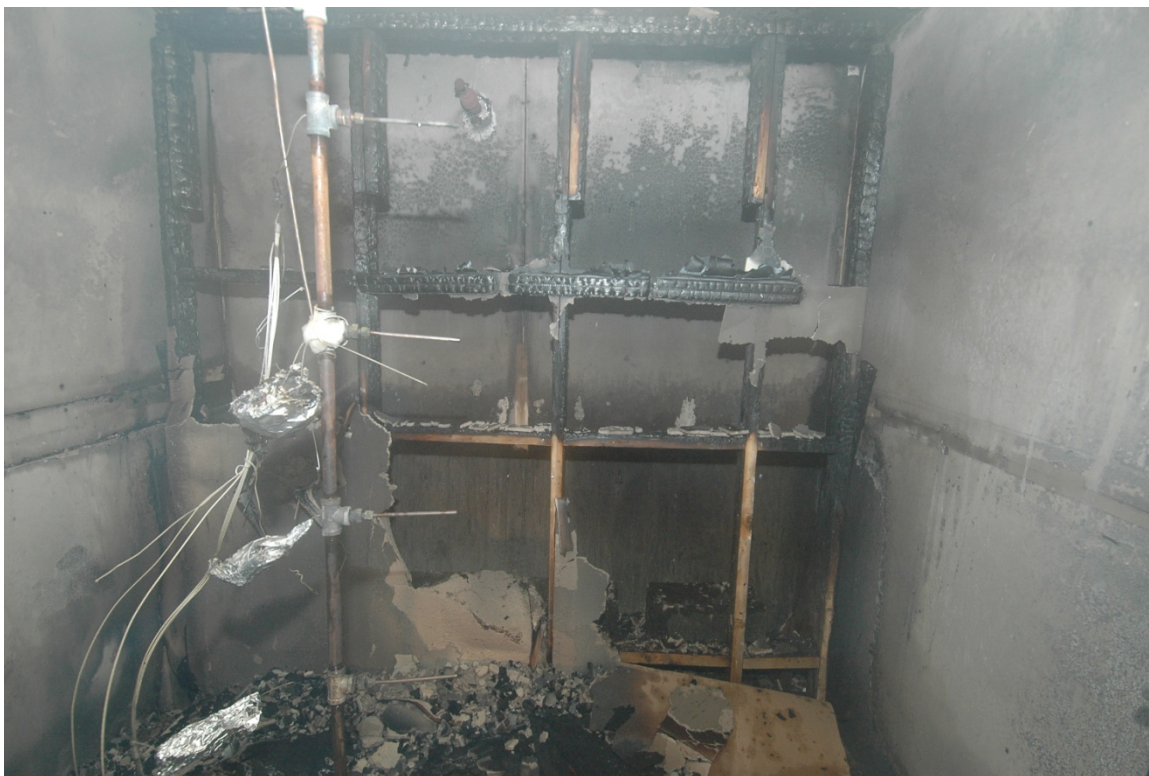
Figure 8-14. Fire pattern of test CH4 (open door)
