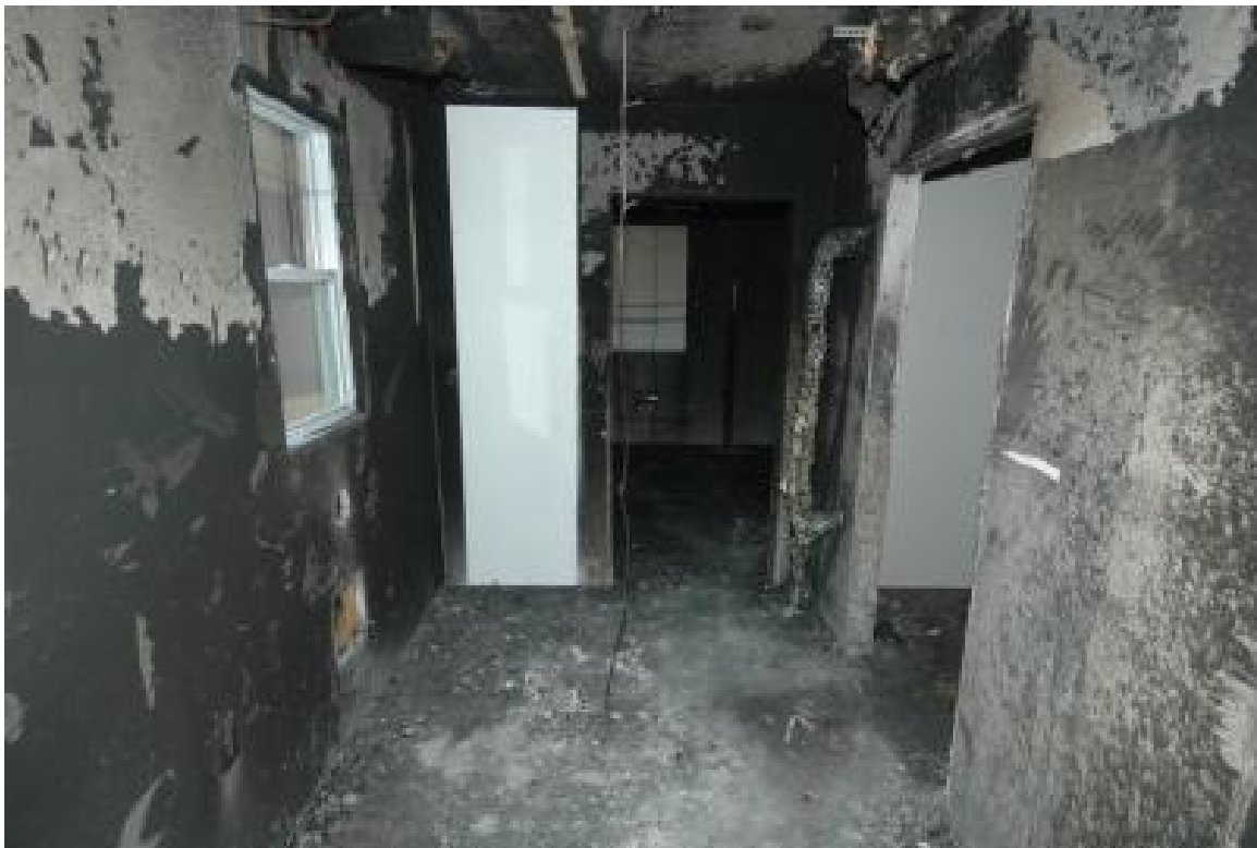
Figure 8-40. Soot deposition on GWB target after smoldering sofa test (SM4 – no ventilation)
