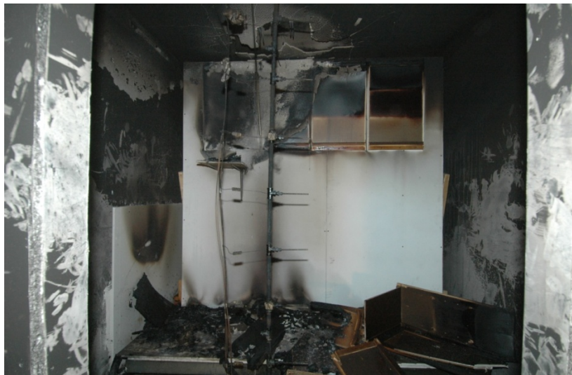
Figure 5-43. Test CH2 damage – high cabinets with half open window
