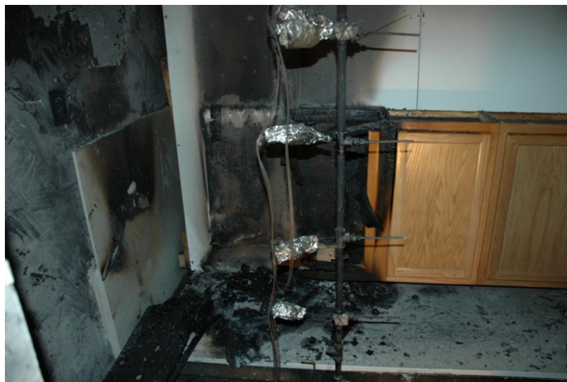
Figure 5-35. Test CL2 damage – low cabinets with half open window
