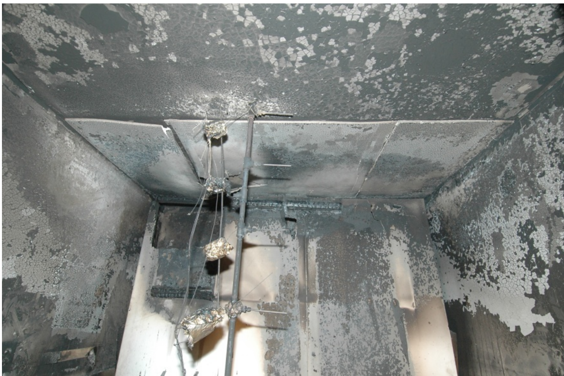
Figure 8-13. Fire pattern from test CH3 (no window)
