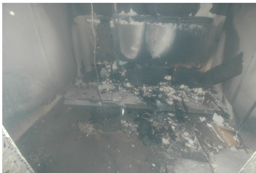
Figure 5-37. Test CL3 damage – Low Cabinets with Open Door
