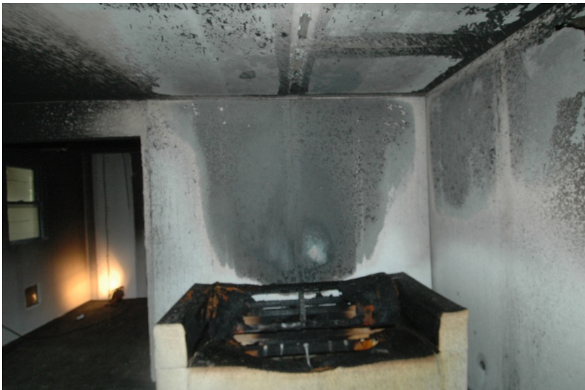
Figure 8-5. Fire pattern from test S2 (full open window)
