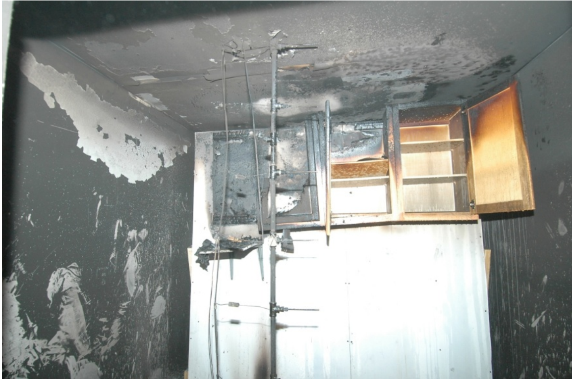
Figure 8-11. Fire pattern from test CH1 (no ventilation)
