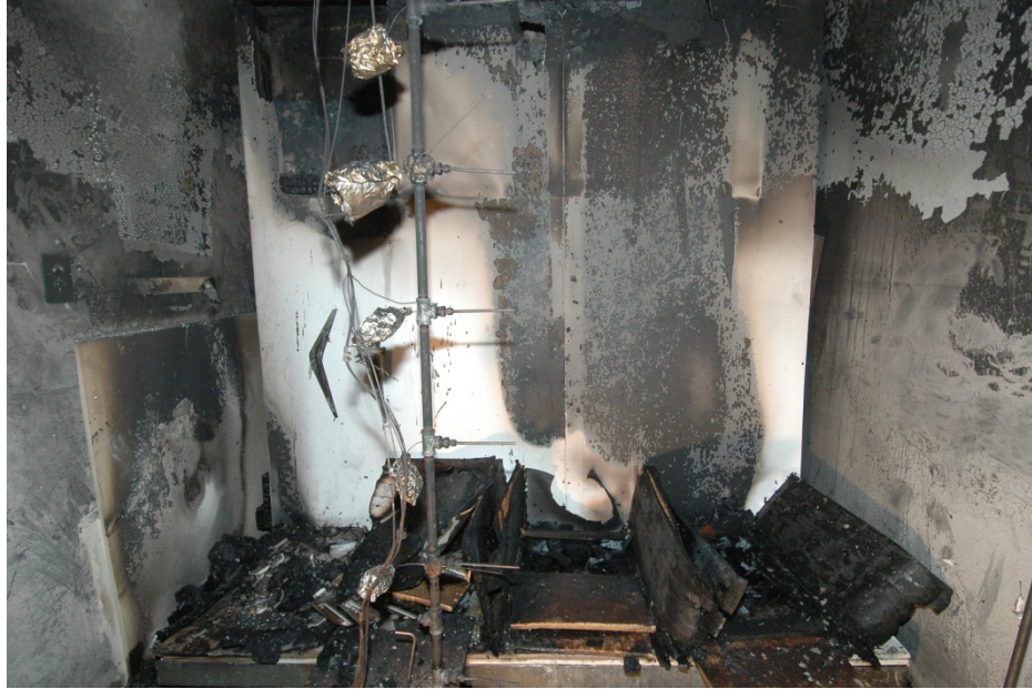
Figure 5-45. Test CH3 damage – high cabinets with no bedroom window
