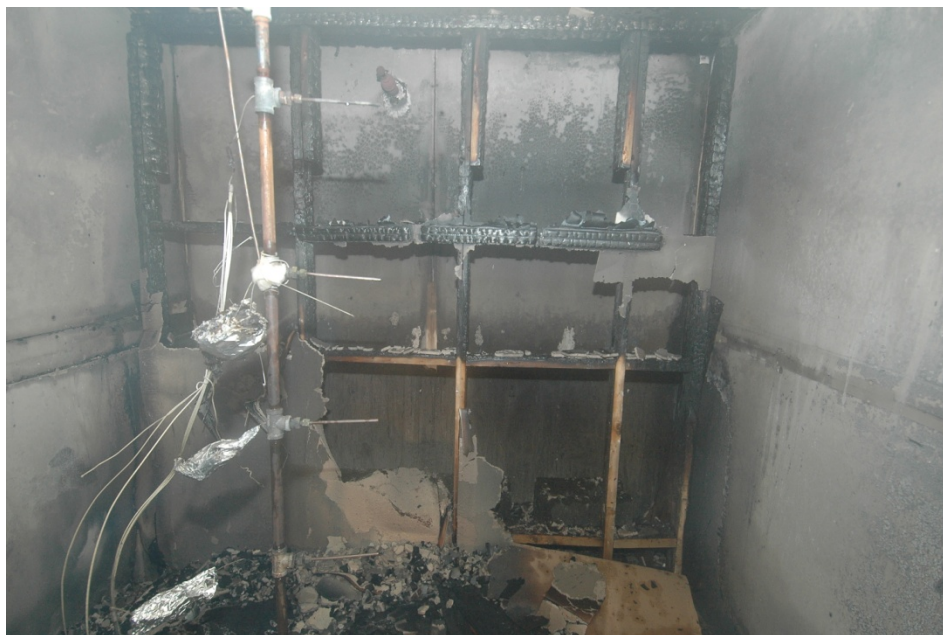
Figure 5-47. Test CH 4 damage – high cabinets open door
