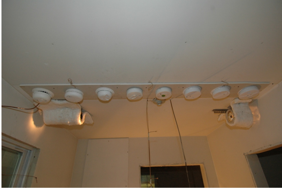
Figure B-3. Photo of smoke alarm array 2
