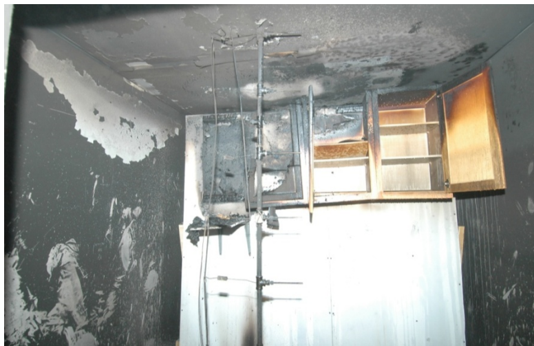
Figure 5-41. Test CH1 damage – high cabinets with no ventilation
