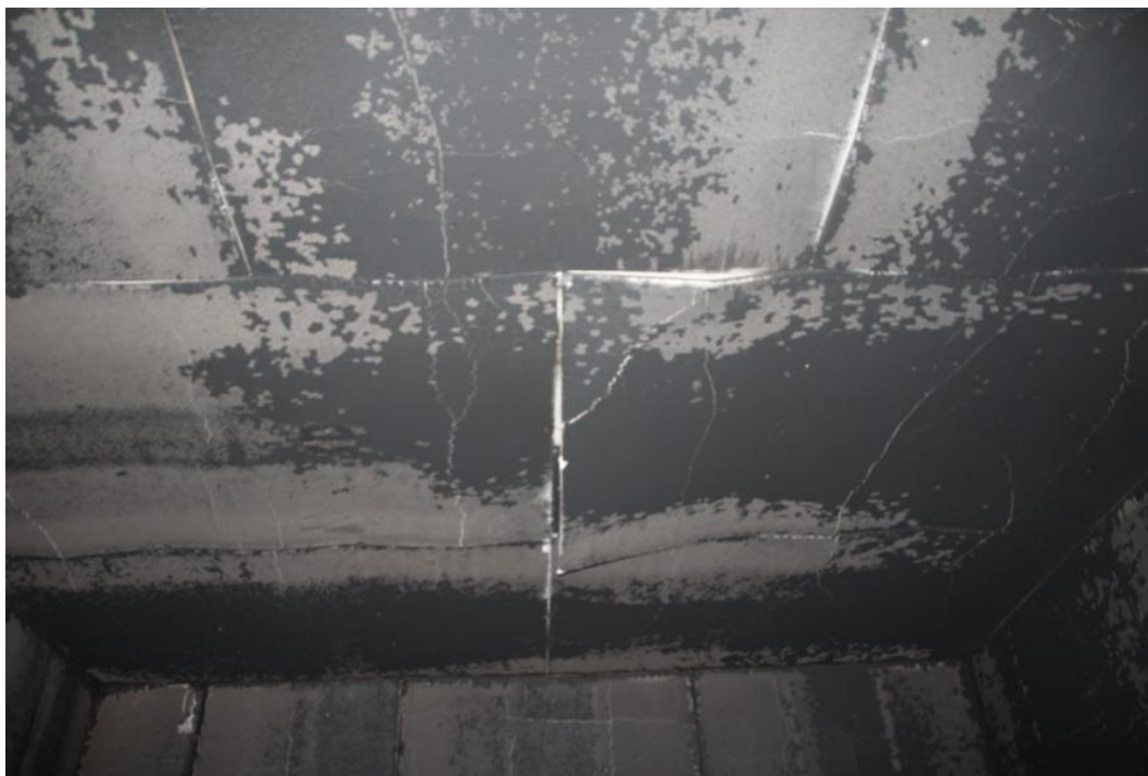
Figure 89. Ceiling of enclosure after Test 6-4.
