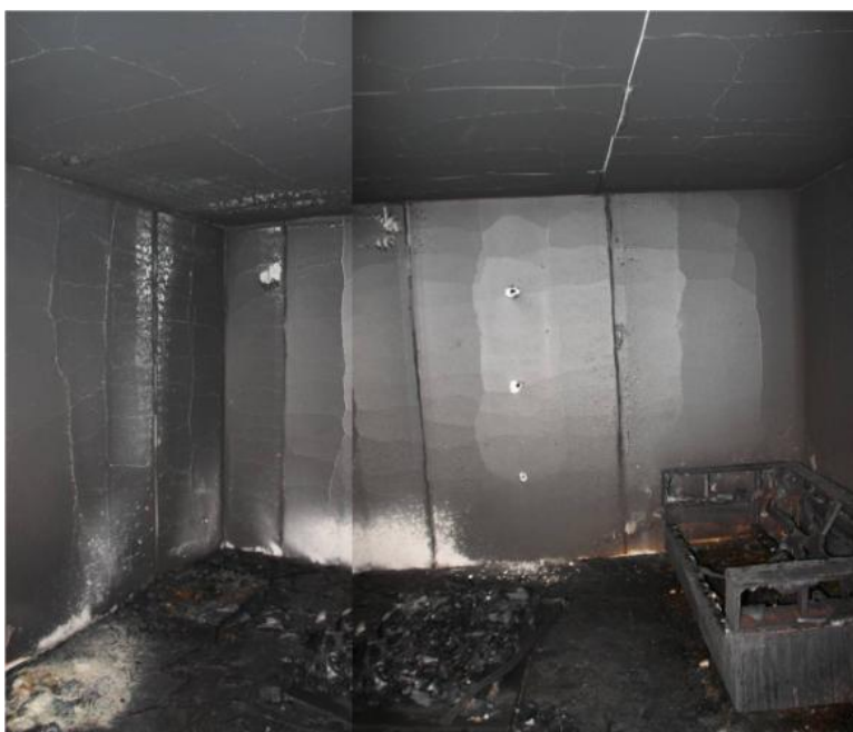
Figure 100. Composite photograph of enclosure conditions after Test 6-6.
