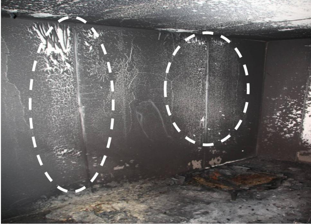
Figure 95. Whitish patterns of relatively reduced soot that were located on the walls above the upholstered chair and baby seat after Test 6-5.
