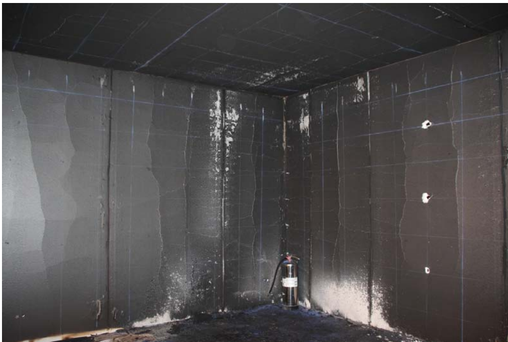
Figure 22. Chalk line grid (blue) installed over top of thermally damaged GWB for calcination depth survey.
