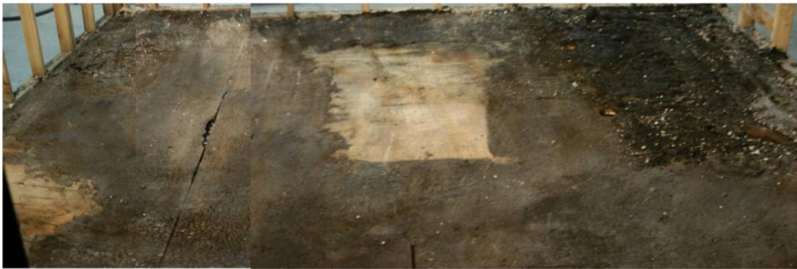
Figure 86. Composite photo of flooring after removal of fire debris from Test 6-3.
