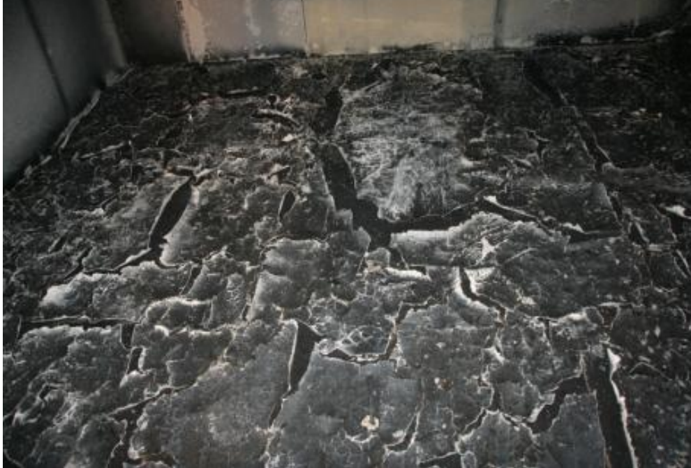
Figure 54. Condition of vinyl flooring after 2.0 L (0.52 gal) gasoline spill fire in enclosure.
