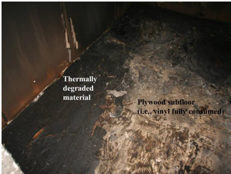
Figure 110. Close up of difference in damage to flooring after Test 6-7.
