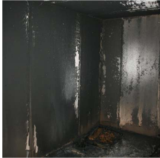
Figure 106. Condition of wall behind upholstered chair after Test 6-7.
