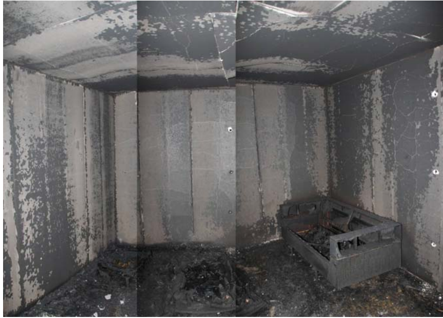
Figure 87. Composite photo of the enclosure after Test 6-4.
