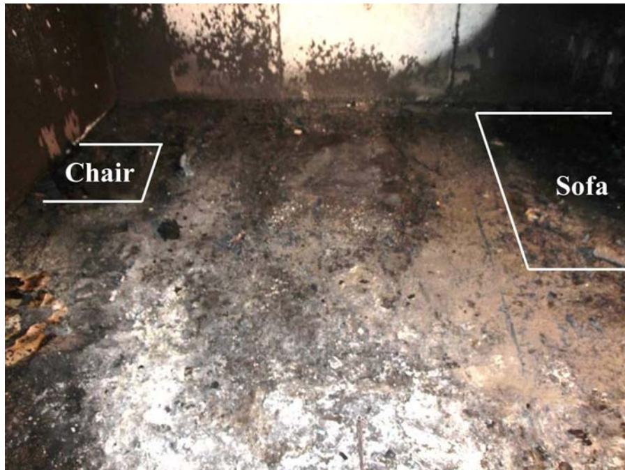
Figure 98. Condition of vinyl flooring after Test 6-5.
