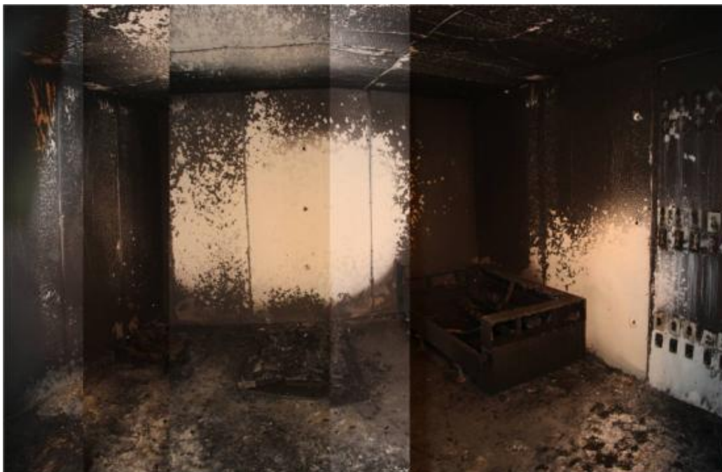
Figure 93. Composite photograph of enclosure conditions after Test 6-5.
