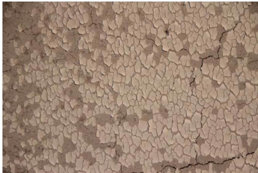
(b). Close up photograph of paper ash on gypsum wallboard.
