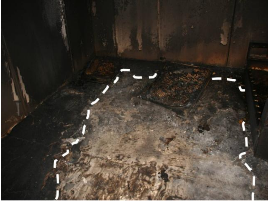
Figure 109. Condition of vinyl flooring after Test 6-7.
