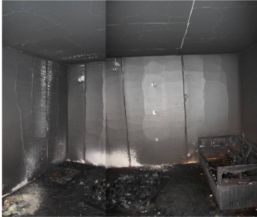
Figure 28. Condition of the walls and ceiling of enclosure after Test 6-6.
