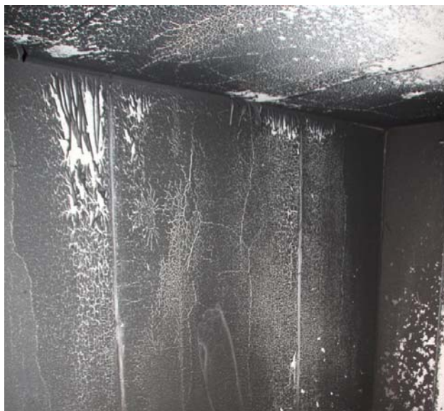
Figure 114. Example of sooted GWB paper that was partially consumed during Test 6-5.
