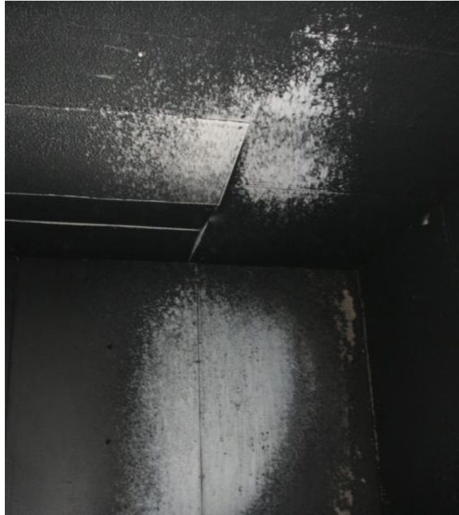
Figure 65. Pattern on ceiling of enclosure after Test 6-1.
