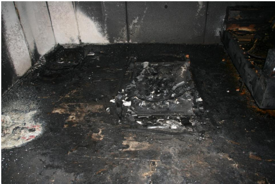
Figure 113. Condition of vinyl flooring after Test 6-8.
