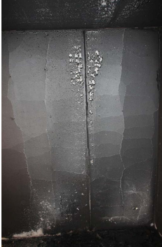
Figure 102. Photograph of absence of soot noted on left wall of the enclosure behind the upholstered chair.
