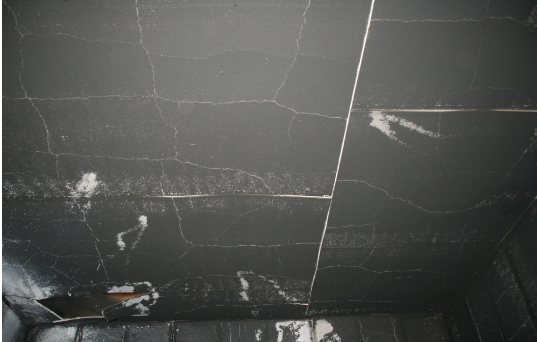
Figure 33. Condition of enclosure ceiling after Test 6-8.
