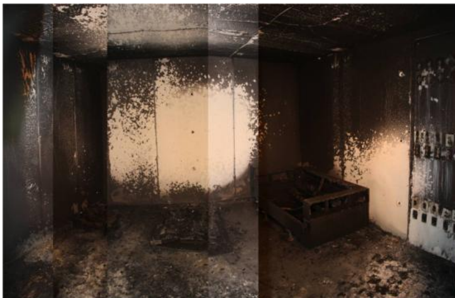
Figure 26. Fire patterns on walls and ceiling of enclosure after Test 6-5.
