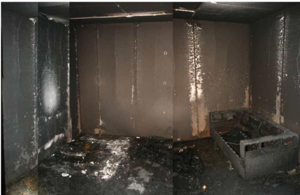
Figure 79. Composite photograph of enclosure conditions after Test 6-3.
