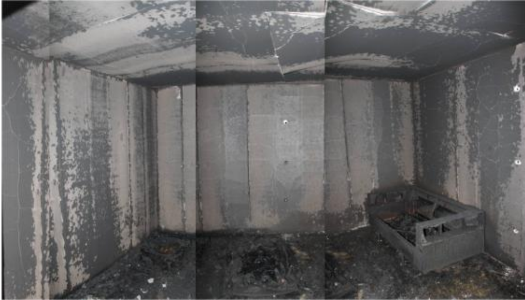
Figure 24. Composite photograph of fire patterns on walls and ceiling of enclosure after Test 6-4.
