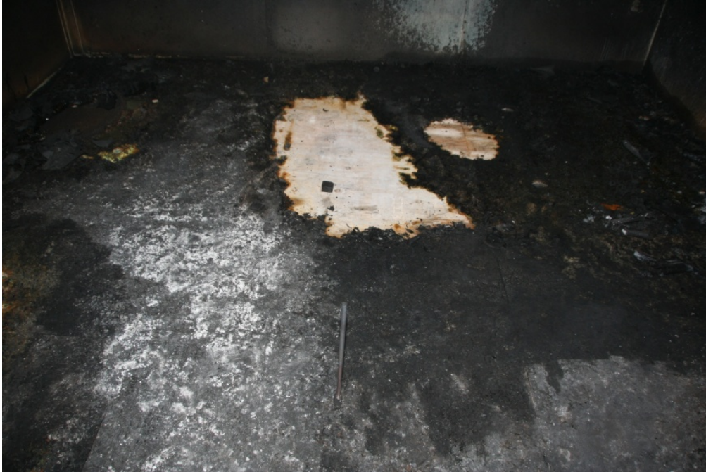
Figure 73. Condition of flooring material after furniture debris cleared from the room in Test 6-1.
