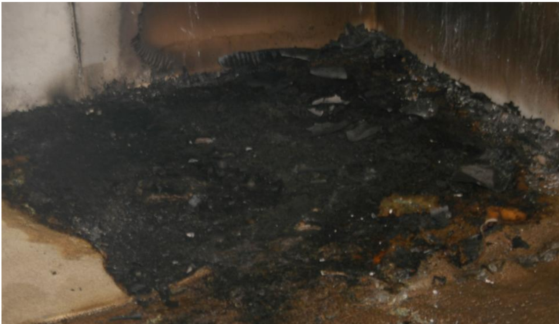
(b) Floor area of initiating spill fire between table and sofa
